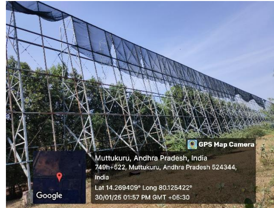
Damaged wind shields towards Krishnapatnam village
