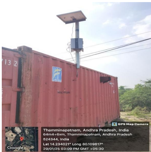
Newly installed CAAQM Station
